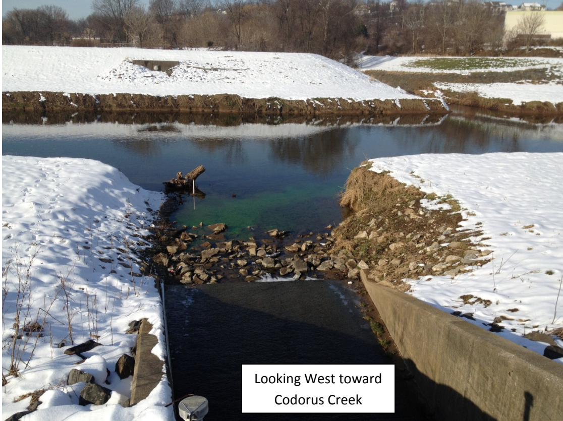
Figure 3.1-33 Fluorescein Dye Seepage into Codorus Creek December 20, 2013
